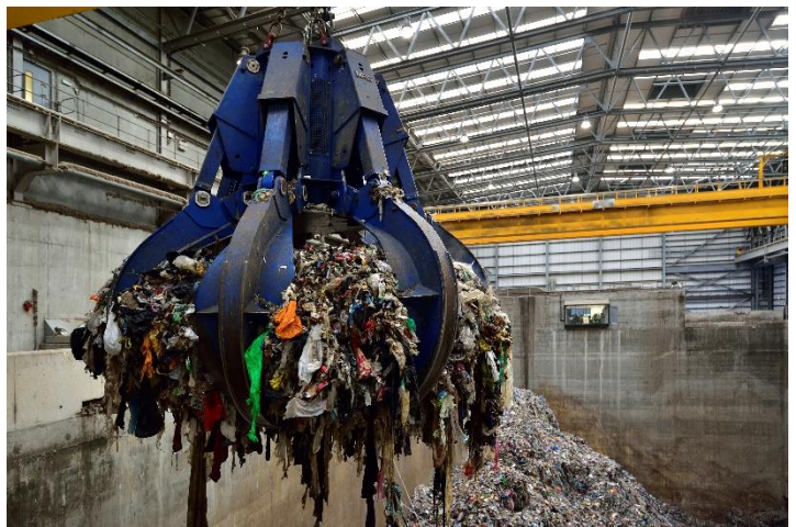
Energy from waste plant
